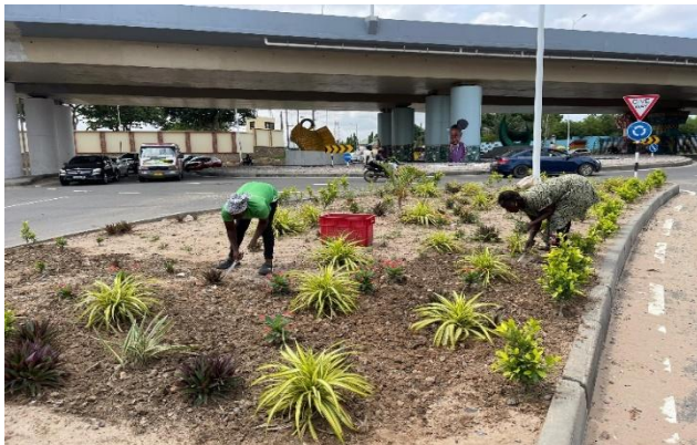
Planting being carried out on the Spintex road median, close to flowerpot.
